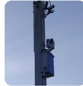
Video surveillance and radar systems
