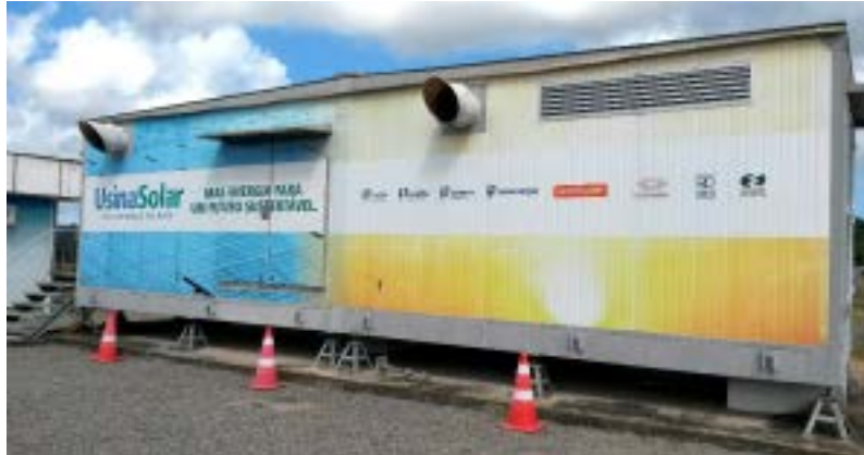
Solarimetric Station installed in Federal University of Pernambuco
