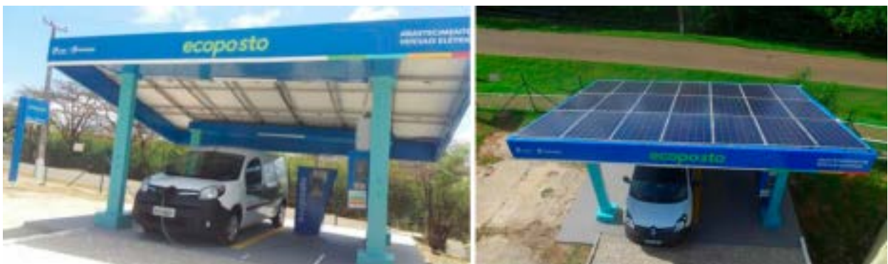
Car electric charging station.
