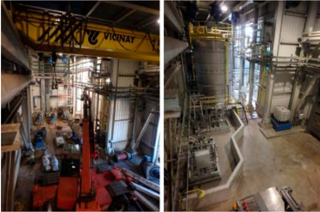
Before and after adapting the desulphurisation building and installing equipment to inject urea into the boiler.
