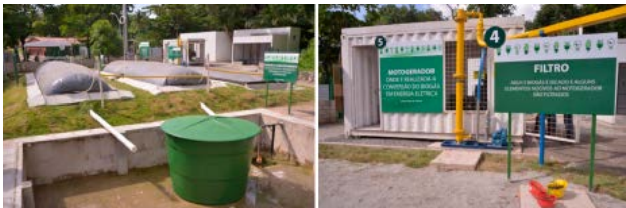
Micro Generation Plant for Biogas from solid waste
