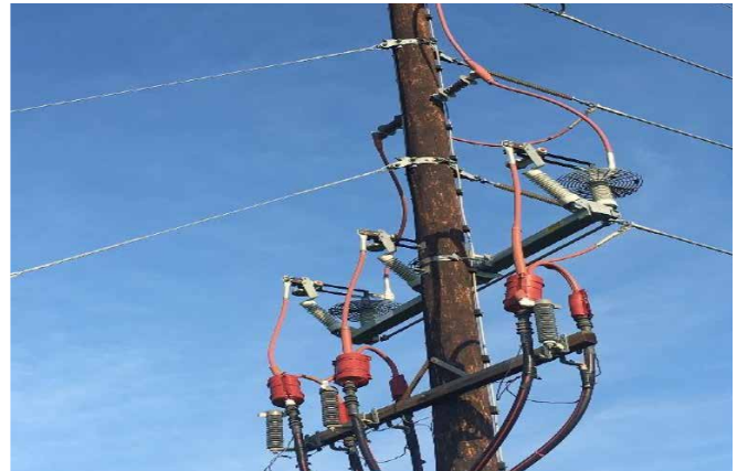
Example of a riser pole with coverings and barriers to minimize risk of wildlife electrocution and resulting plant outage.
