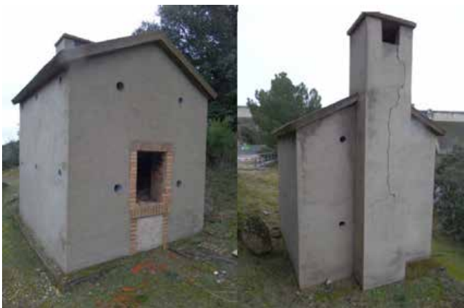
Generation plant burner Agavanzal
