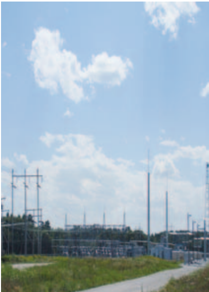
Electrical substation Maine (USA).
