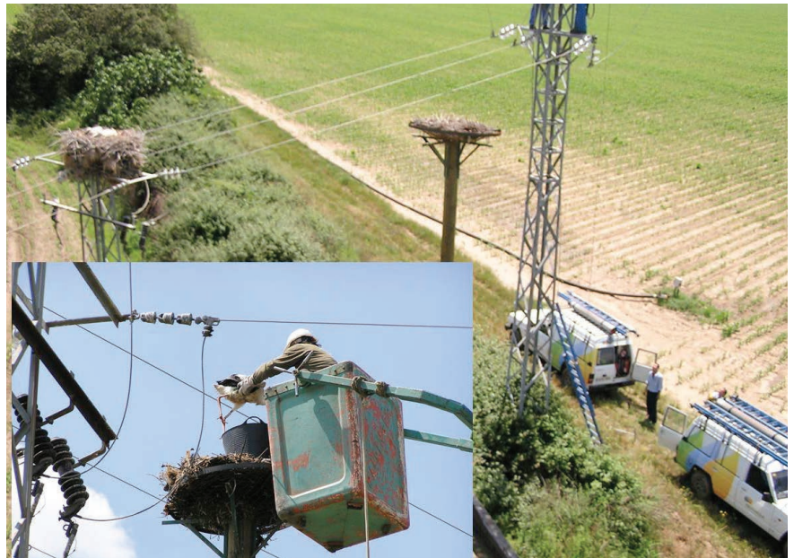
Relocating stork nests from power lines in Extremadura
