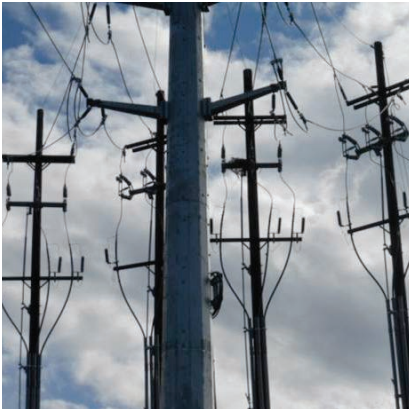
Electricity pylons, USA
