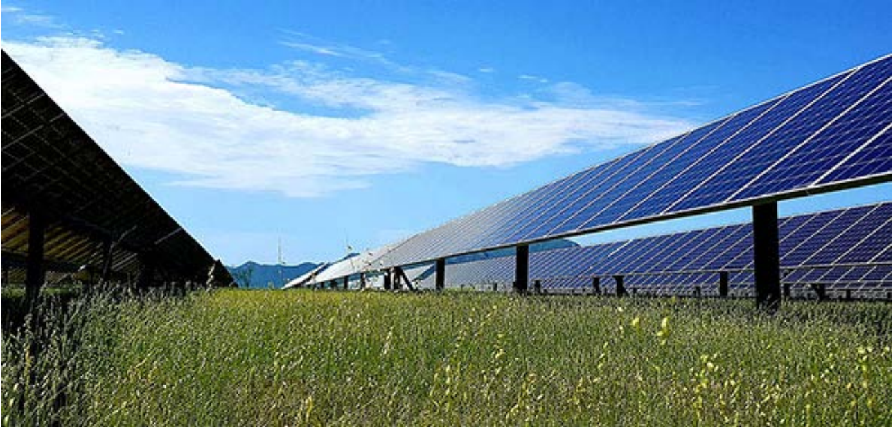
Hermsillo solar photovoltaic power plant - Sonora, Mexico
